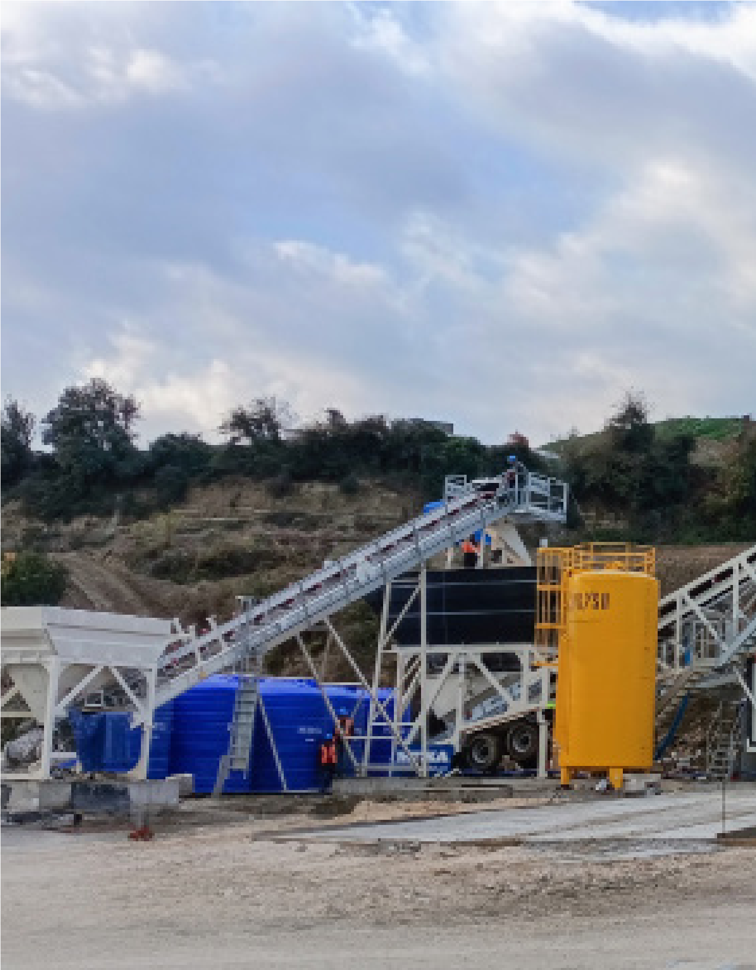
▲ MEKA Mobil Beton Santrali Hatay
